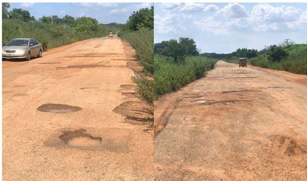
Fig. 2b. Photos showing parts of the road with failed pavement
