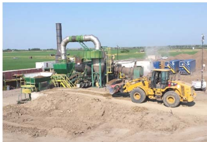
Direct fired thermal desorption unit
