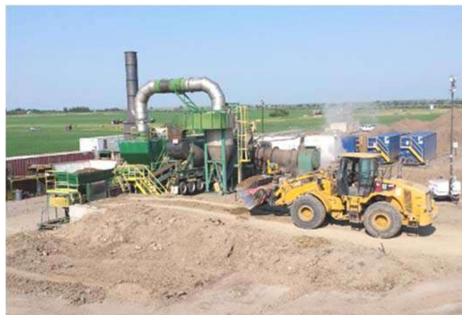
Direct fired thermal desorption unit
